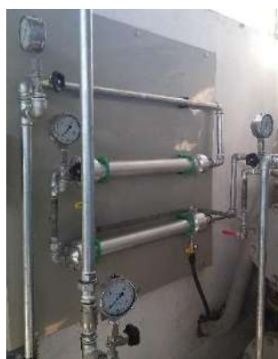
Figure 1. Two-stage membrane separation unit for biogas upgrading.
